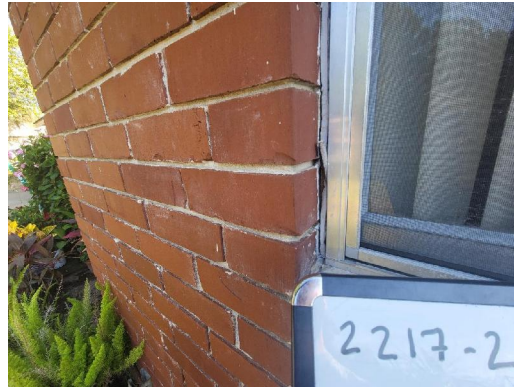
2217-2 Caulk/Glazing/Off-White Typical Exterior Windows 4% Chrysotile
